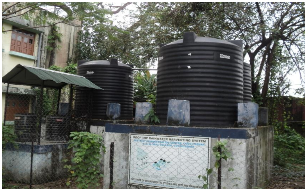
Photograph No.7.1: The Roof Top Rain Water Harvesting System
